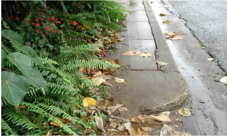
Figure 5: 'Poorly maintained footpath'
